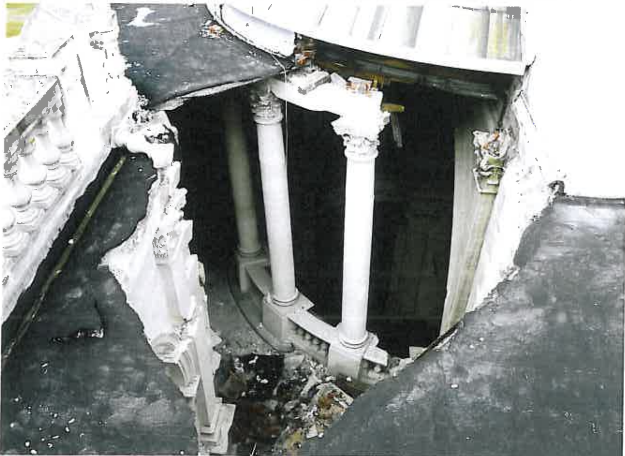
Looking through the collapsed roof into the interior of the cathedral beneath the main dome. Image courtesy of Opus International Consultants
