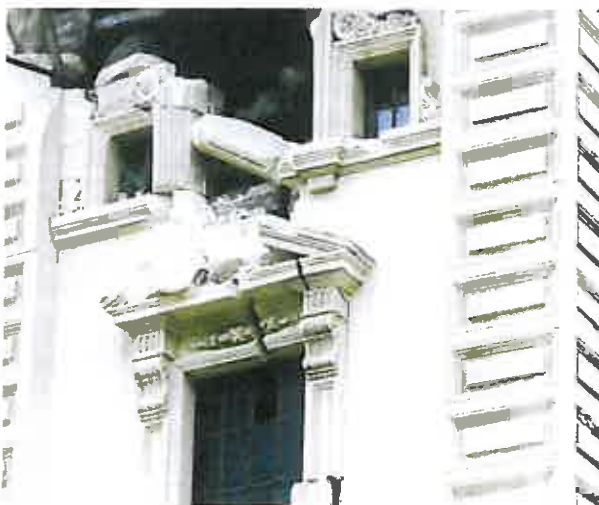
Some of the work to protect and to completely restore the basilica is already well under way. Image courtesy of Opus International Consultants
