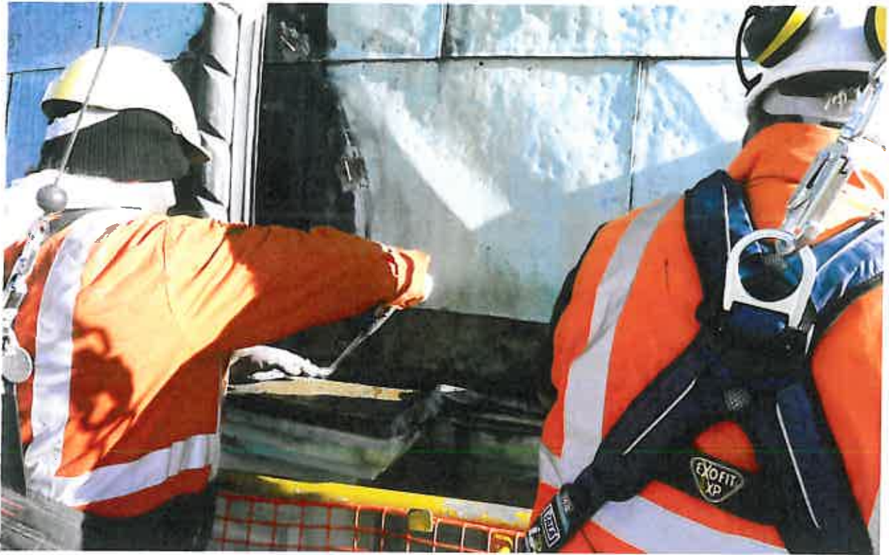
Images: In the team: Duayne Vercoe Crane Driver/Dognan and Murray Flett Site Manager, complete preparations for removing the stonemason's dome. Image courtesy of Goud International Consultants
