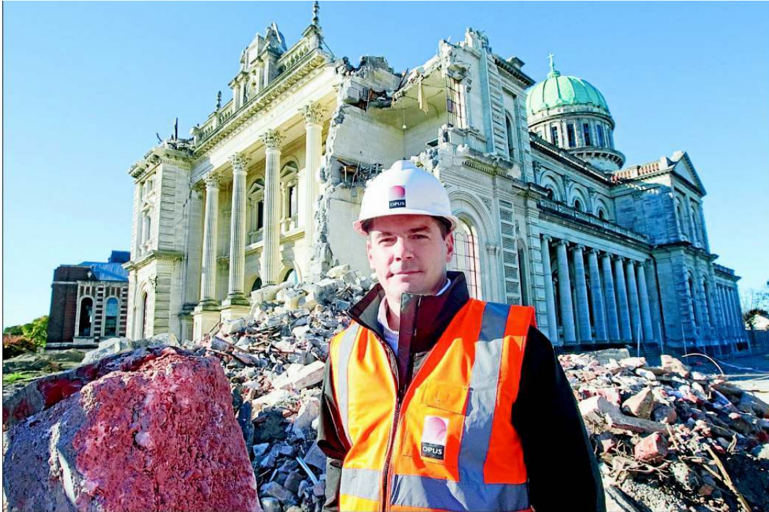
Big jobs: Opus heritage and structural engineering experts are deconstructing the unstable north tower in Christchurch's Catholic Cathedral and also plan to remove the building's main dome. The aim is to stabilise the cathedral so the damage can be thoroughly assessed and a fully informed decision as to the future of the building can be made. Photo: THE PRESS
